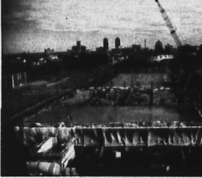
A bird's eye view of the construction on Phase II of the Science, Engineering and Technology complex shows progress made so far. Expected completion is sometime this summer. Photo by JOHN HERNANDEZ
