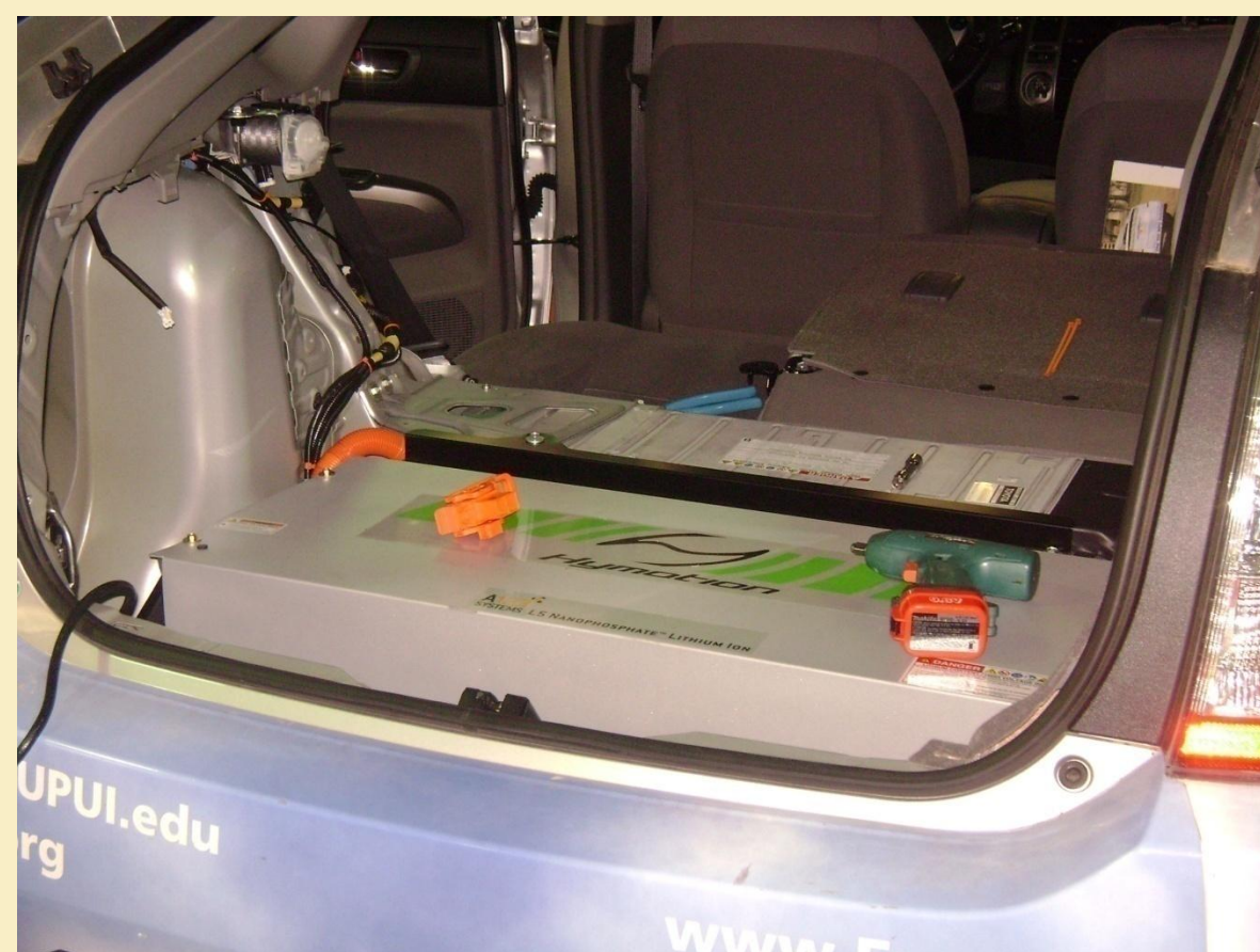
Fig 2: 5 Kwh Li-Ion battery installed.
