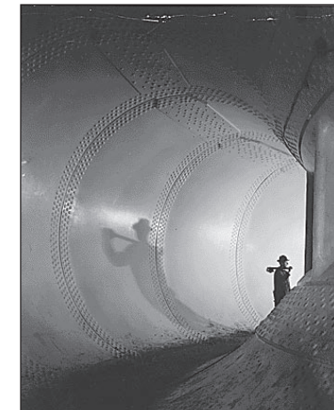
A Tennessee Valley Authority hydroelectric dam under construction. Courtesy of Franklin D. Roosevelt Library.
